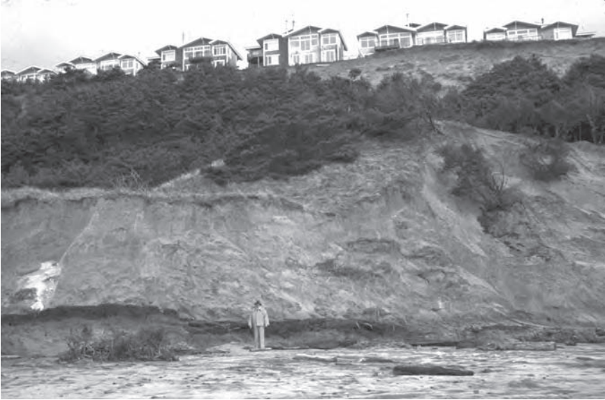
Figure CS9.5 The toe (foreground) of the landslide and its slip face in front of The Capes condominiums (1999)
