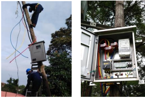
Fig 5: GSM – Based post – paid smart meters being installed.
