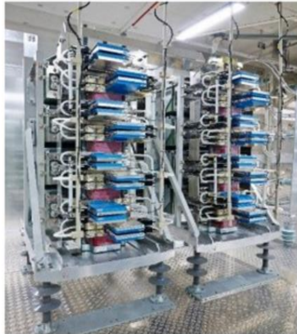
Fig.1b A photo of installed MOS-FET Source: ABB- An introduction to Facts- 2006
