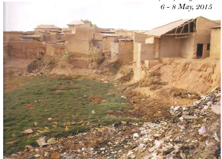
Fig. 6: Collapsed walls of houses close to Ramin Masu pond at Gafai quarters.
