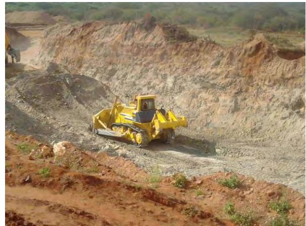
Figure 4 a bulldozer pushing loose material and developing bench and access to rich iron vein.
